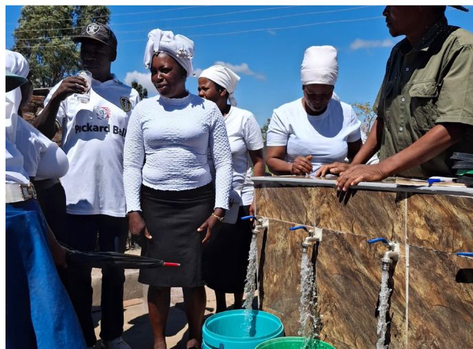
Solar-powered borehole installed and fully operational – supplying approximately 3,000 people.
